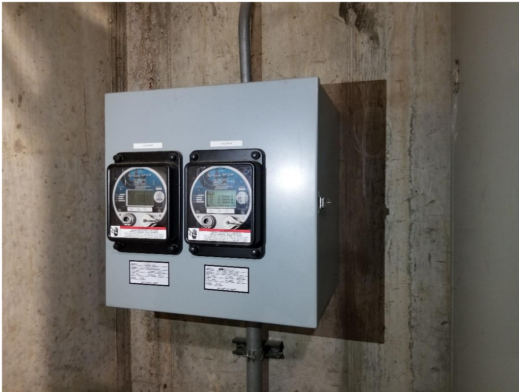
Installed Nexus® 1272 Power Quality Meters
