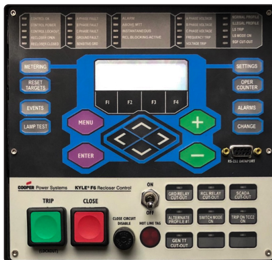
Figure 3 Verify that Eaton Cooper Form 6 Control is Powered OFF
