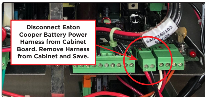
Figure 16 Eaton Cooper Battery Power Harness - Cabinet Board Location
