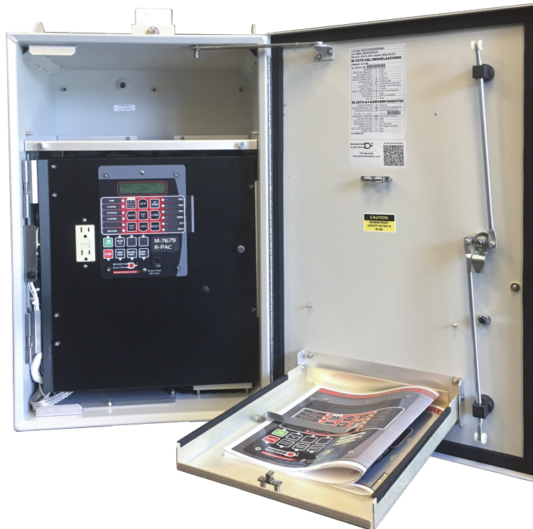
Figure 3 M-2979 Recloser Control Cabinet
